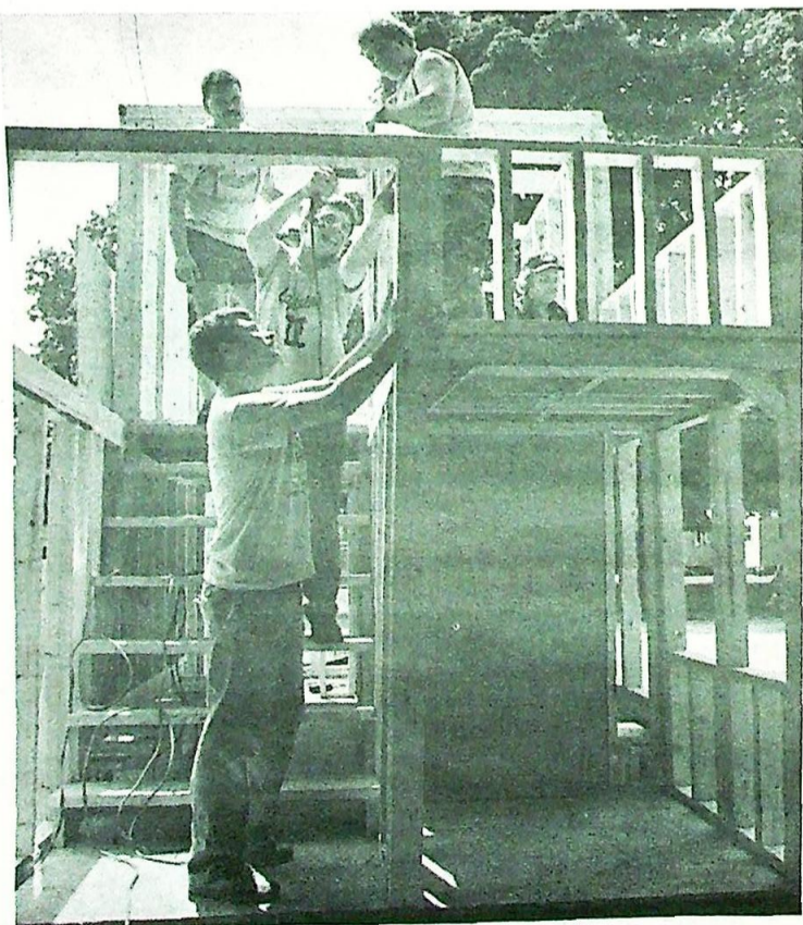
Members from area V.F.D. (District 3) work on the frame work of the "EDITH" House or Fire Safety House. KKK Vol. F.D.
