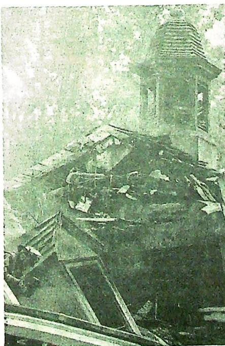
By Randy Greenwell A firefighter douses hot spots in Oak Meadow clubhouse rubble.
