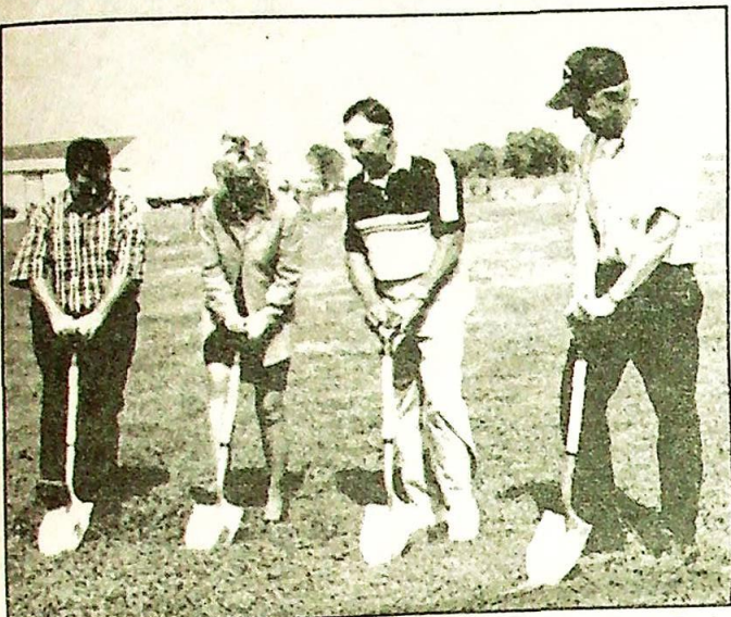
Left to right: Ed Flynn - Hamilton Twp. Board President, Becky Skillman, Indiana State Senator, Kenny Runge and Howard Wentte, contractors. (Photo submitted by Donald Schnitker)
