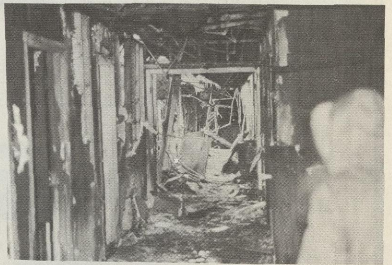
Looking down main corridor towards Sanctuary, the "muddy" looking floor is from the ceiling tile that had fallen and gotten wet. On the left, almost to the end of the hall is the furnace room.
