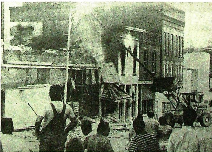
Nearly 300 residents of Williamsport turned out Wednesday afternoon to watch as Jimmy Taylor of Attica knocked down some burned-out downtown buildings. A fire Monday morning destroyed the town's only hardware store, a beauty shop, a barber shop, the offices of two lawyers and the offices of the Warren County school corporation, all in a block of North Monroe Street.
