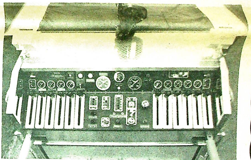
Top controlled operator's panel with color coding of all inlets and discharges
