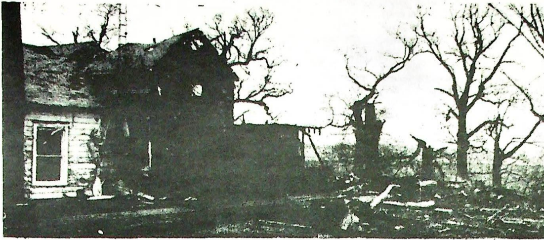
A fire caused extensive damage to this Colfax Township home of Ronald and Dawn Christenson. The fire apparently started in the garage. That is now rubble shown on the right.
