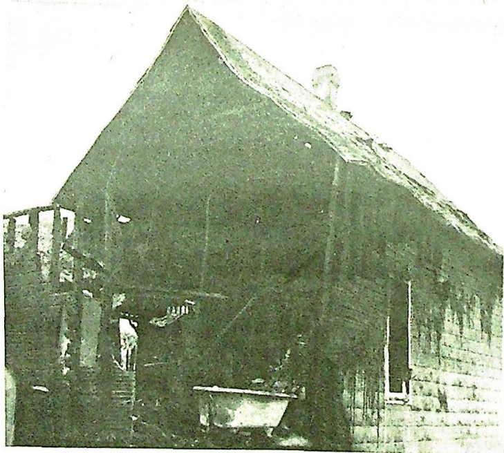
The damage caused by the fatal fire can be seen clearly in this view looking south east. The arrows indicate the upstairs bedroom where the children and grandmother had been sleeping.
